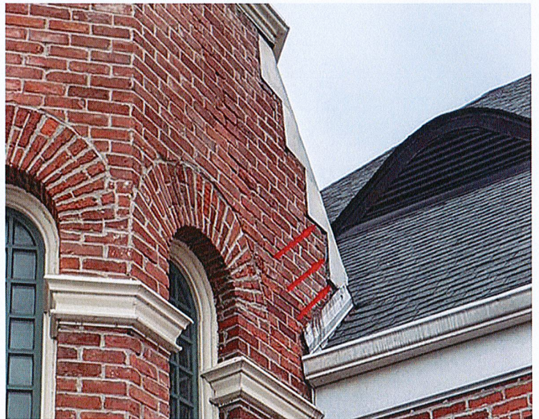
Photo 3 Showing sheet metal cap on tower with large gaps in the mortar joints where the caps are embedded into the masonry. Large open gaps will be repointed and all joints at the embedment areas will receive backer rod and silicone joint sealant.
