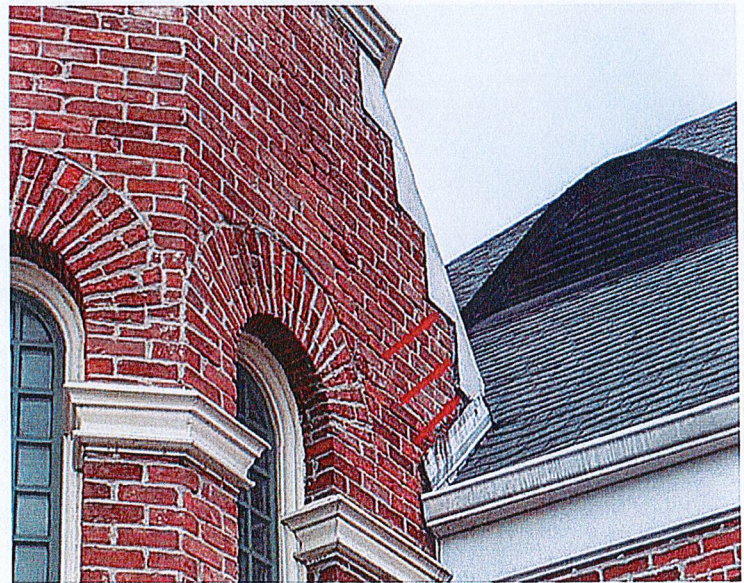
Photo 3 Showing sheet metal cap on tower with large gaps in the mortar joints where the caps are embedded into the masonry. Large open gaps will be repointed and all joints at the embedment areas will receive backer rod and silicone joint sealant.
